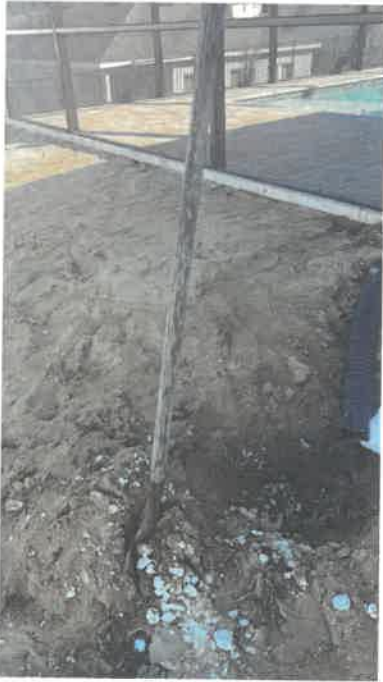
Photos 4 & 5. Water coming from gutters making a hole (on side of pool in construction).
