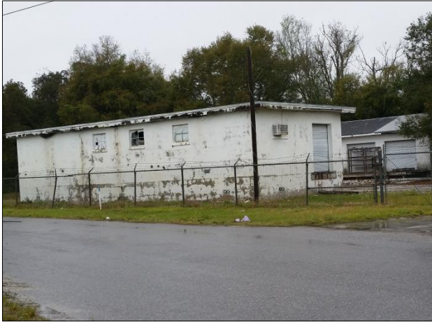
Deteriorated industrial structure
