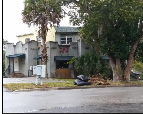
Deteriorated multi-family structure
