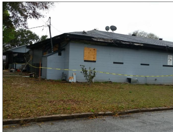
Deteriorating commercial structure
