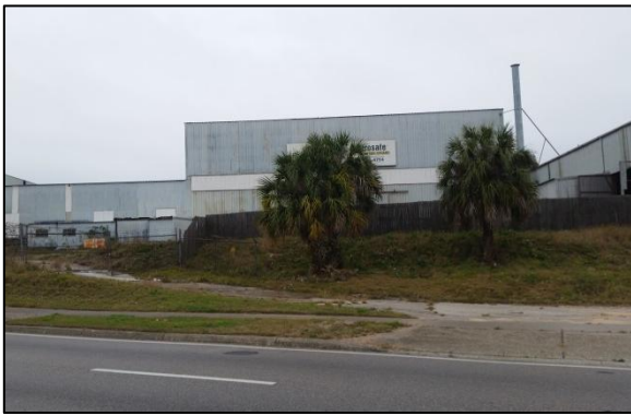
Overgrown landscaping & cracked pavement
