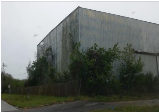
Overgrown landscaping & dilapidated fencing
