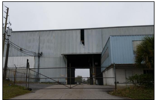
Neglected building damage
