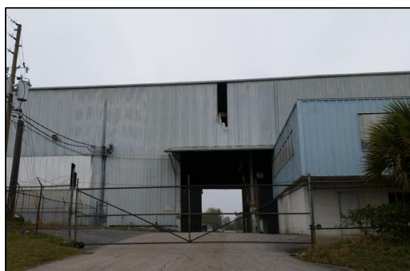
Neglected building damage
