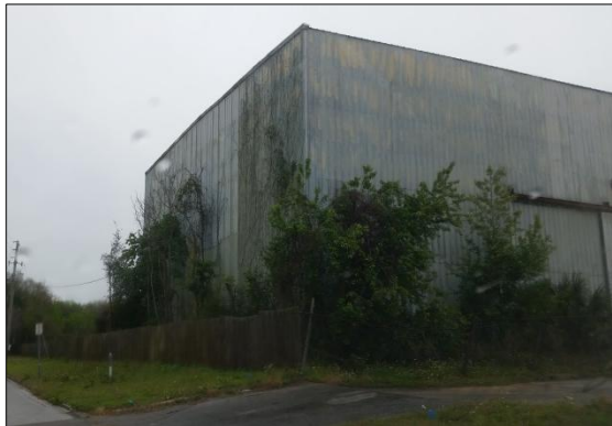
Overgrown landscaping & dilapidated fencing
