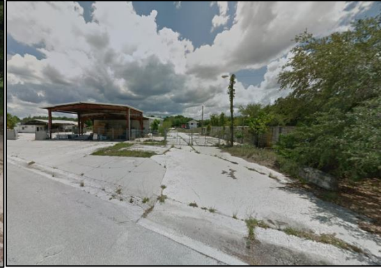
Cracked & excessive paving/driveway
