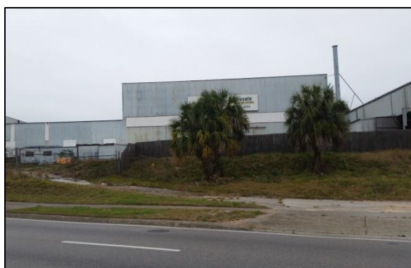
Overgrown landscaping & cracked pavement
