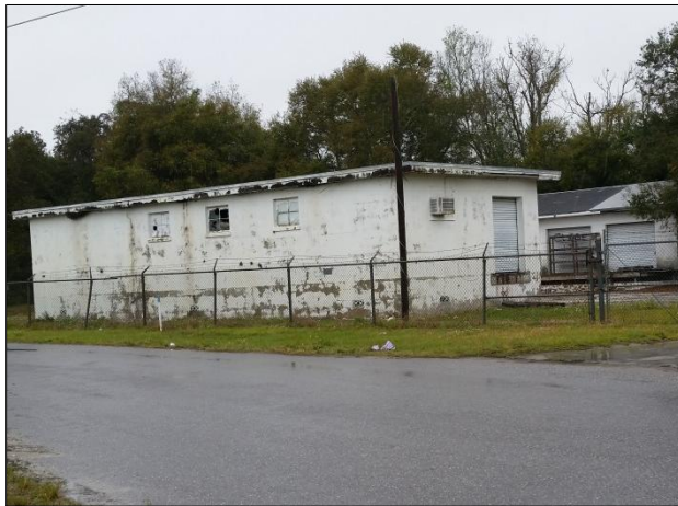
Deteriorated industrial structure
