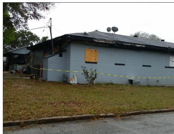
Deteriorating commercial structure
