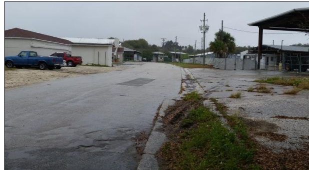
Cracked overgrown driveways & dirt driveways
