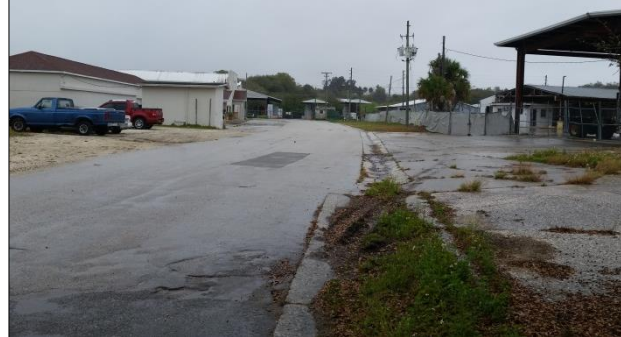
Cracked overgrown driveways & dirt driveways
