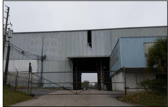
Neglected building damage
