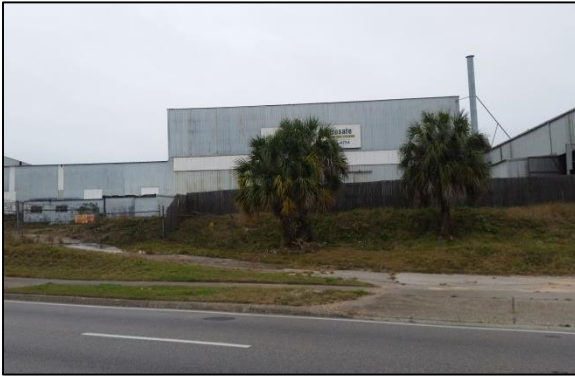
Overgrown landscaping & cracked pavement
