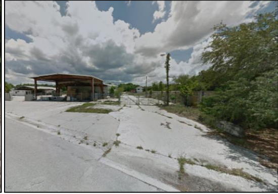
Cracked & excessive paving/driveway
