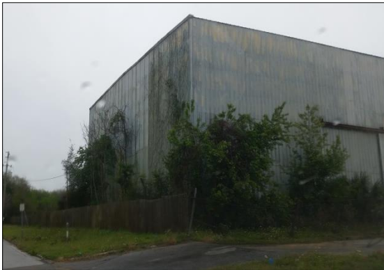
Overgrown landscaping & dilapidated fencing
