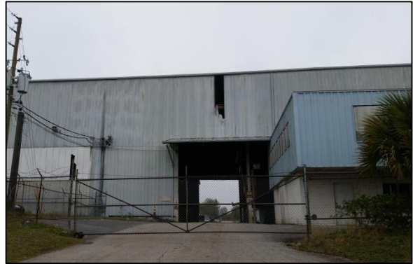
Neglected building damage
