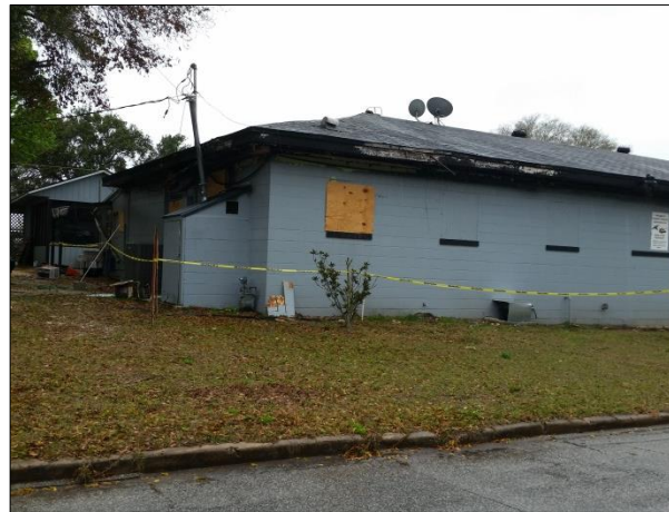
Deteriorating commercial structure
