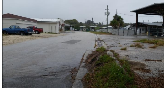
Cracked overgrown driveways & dirt driveways
