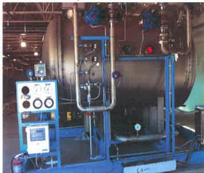
Fuji Ozone Generator
