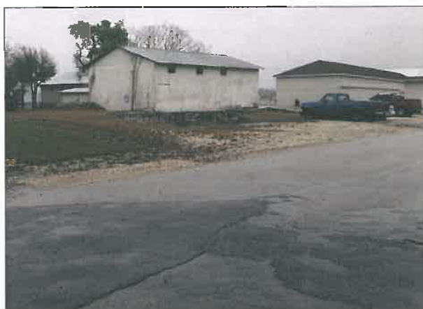
Deteriorated road, lack of curb, gutter & sidewalk
