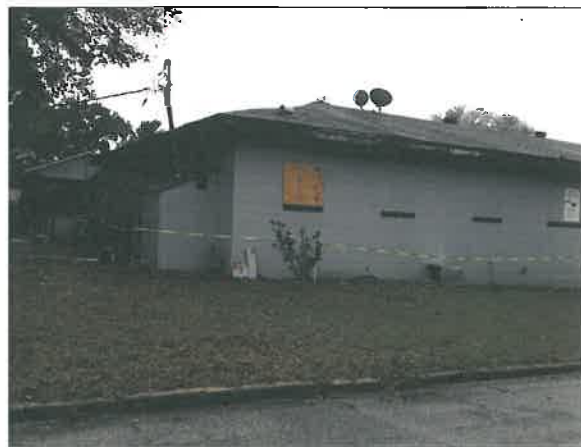
Deteriorating commercial structure
