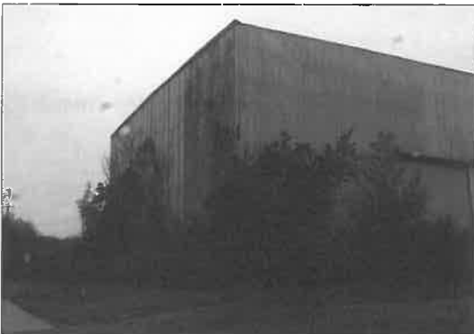
Overgrown landscaping & dilapidated fencing
