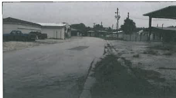
Cracked overgrown driveways & dirt driveways
