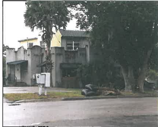
Deteriorated multi-family structure
