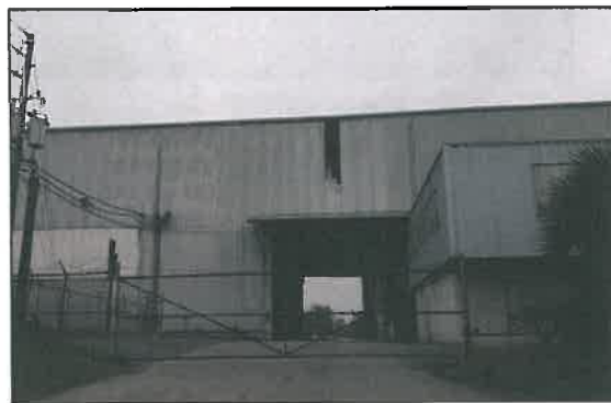
Neglected building damage
