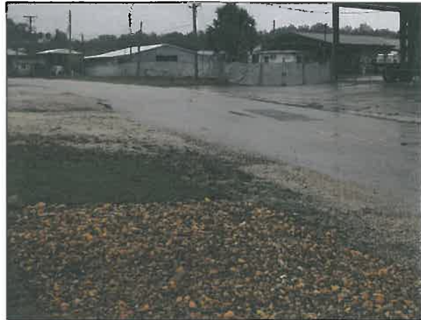
Sand & gravel driveways overflowing into right-of-way
