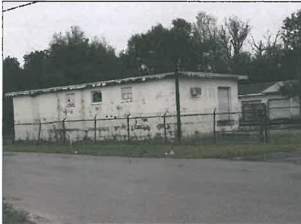
Deteriorated industrial structure
