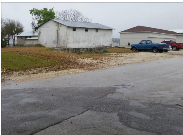
Deteriorated road, lack of curb, gutter & sidewalk
