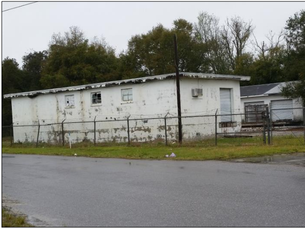
Deteriorated industrial structure
