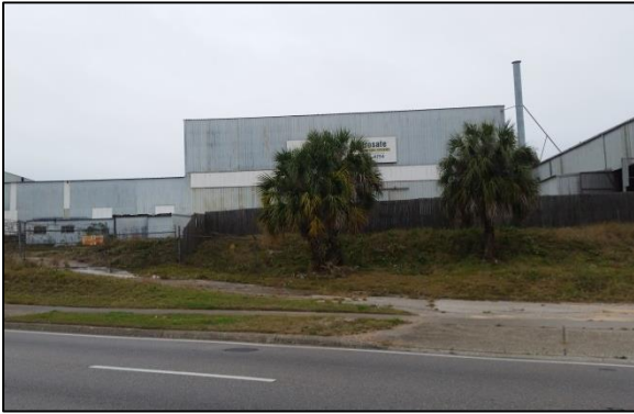
Overgrown landscaping & cracked pavement
