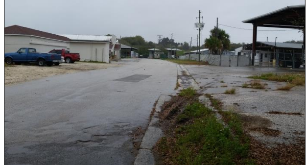
Cracked overgrown driveways & dirt driveways
