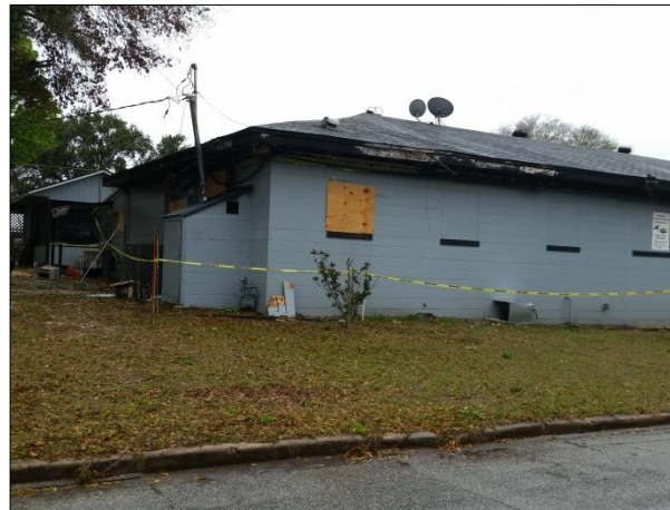
Deteriorating commercial structure
